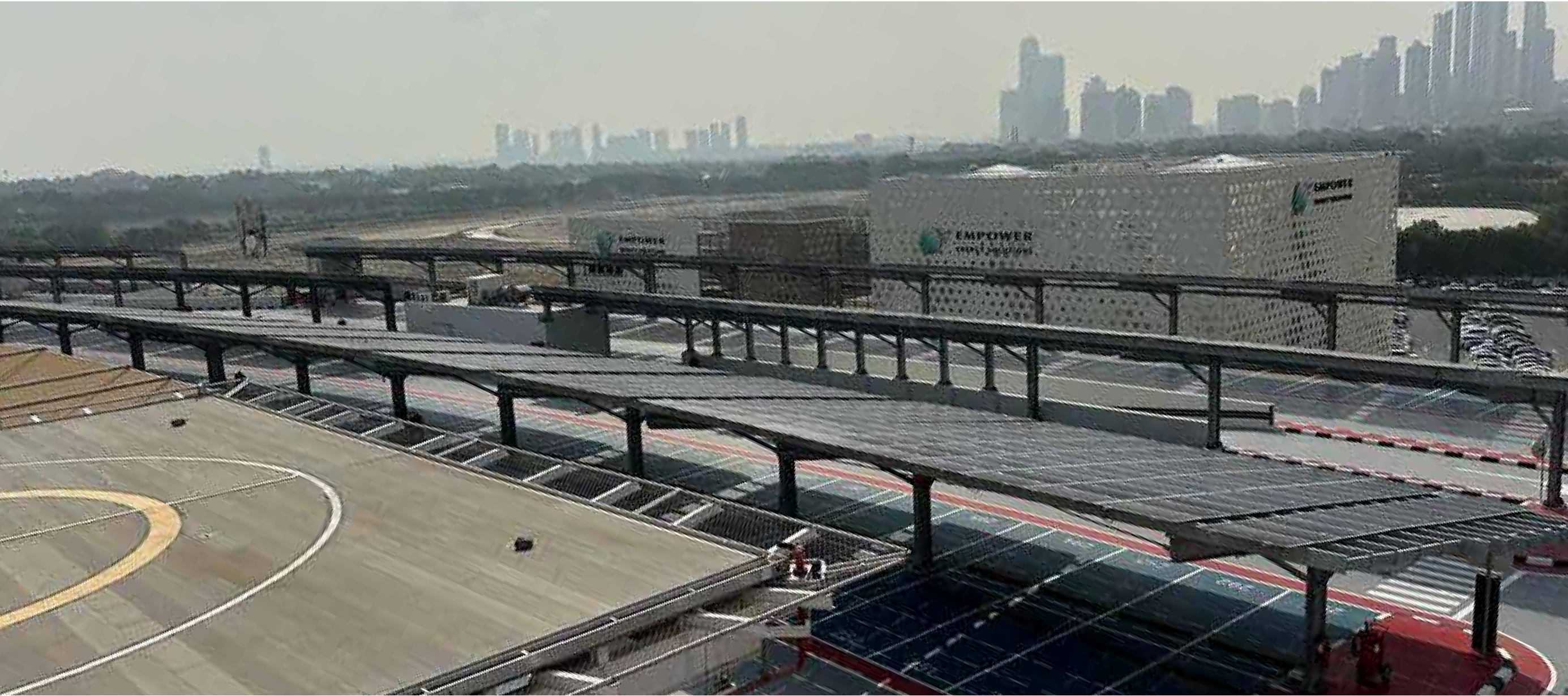
Al-Mustaqbal rooftop solar panels
